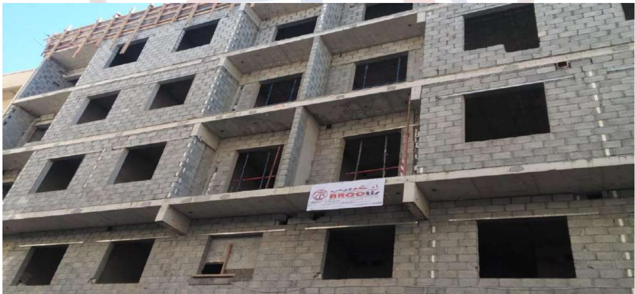
M/s. Falcon Building Contracting, (G+6) Building at Bur Dubai, ARCotis Brand , M.R Passenger Elevators, Speed : 1.0 (m/s), Capacity: 630 KG/8persons.
