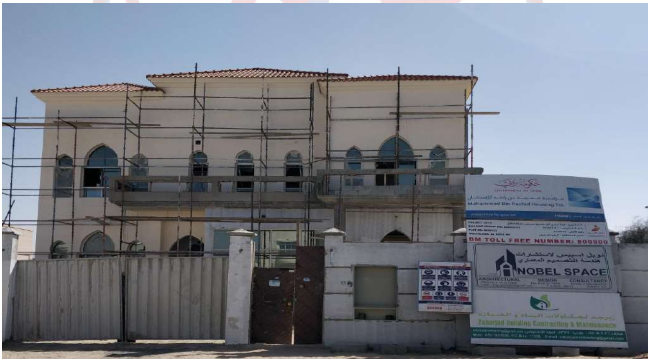
M/s. Nobel Space (G+1) Villa at Dubai, ARCOTIS Brand , MRL Passenger Elevators, Speed: 1.0 (m/s), Capacity: 320 KG/4persons.
